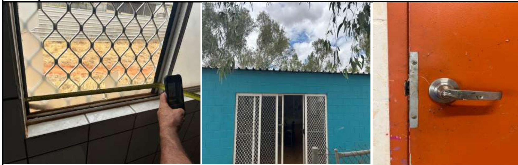
Photos Showing Current Condition of Art Centre:
