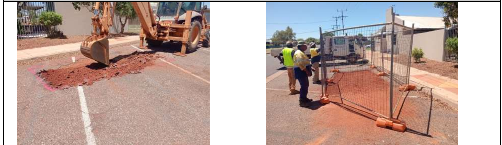
Photos: Existing Potholes
