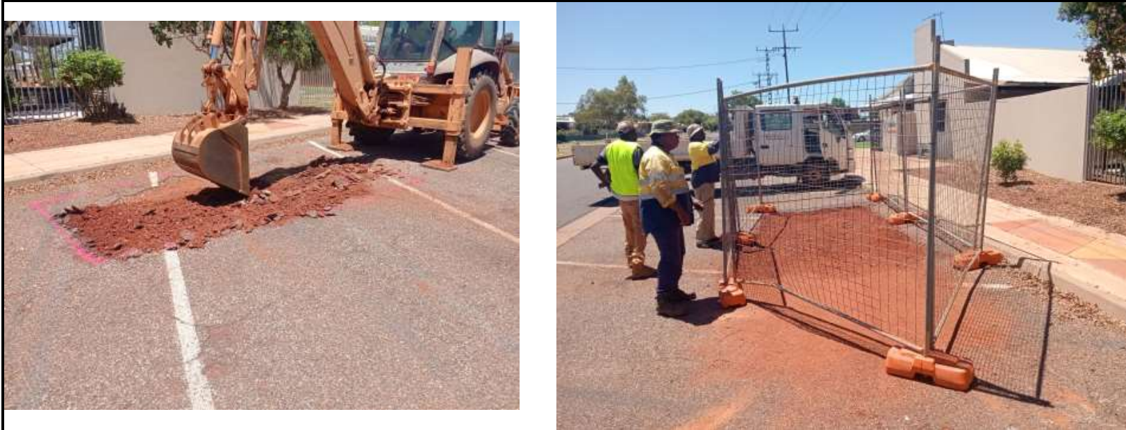
Photos: Existing Potholes
