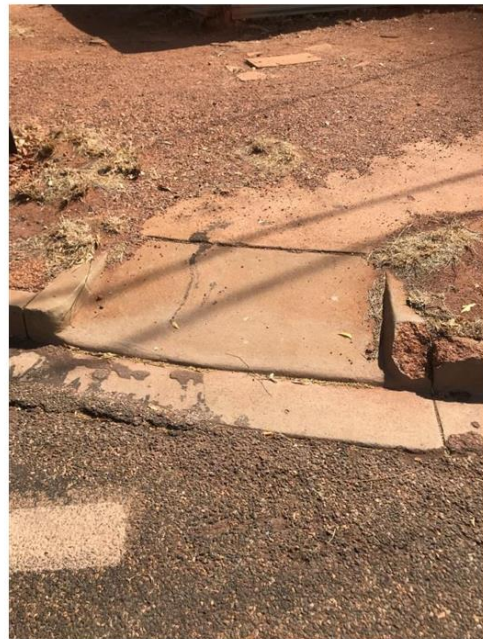
Point 16: Cat 1, reconstruct kerb ramp to size, shape, alignment and slope
