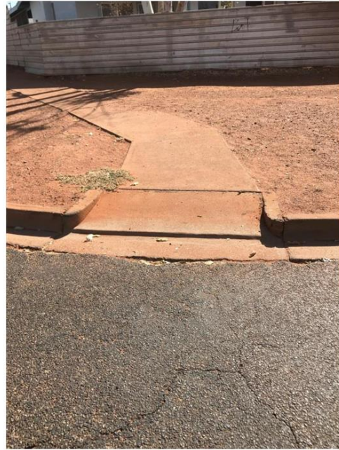
Point 11: Cat 1, reconstruct kerb ramp to size, shape and slope
