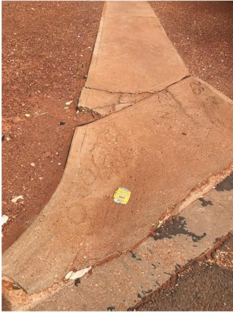
Point 25 : Cat 1, reconstruct kerb to size, shape, alignment and slope
