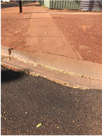
Point 5: Cat 1, reconstruct kerb ramp to shape, size, slope and to the alignment
