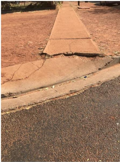
Point 6: Cat 1, reconstruct kerb ramp to shape, size, slope and to the alignment
