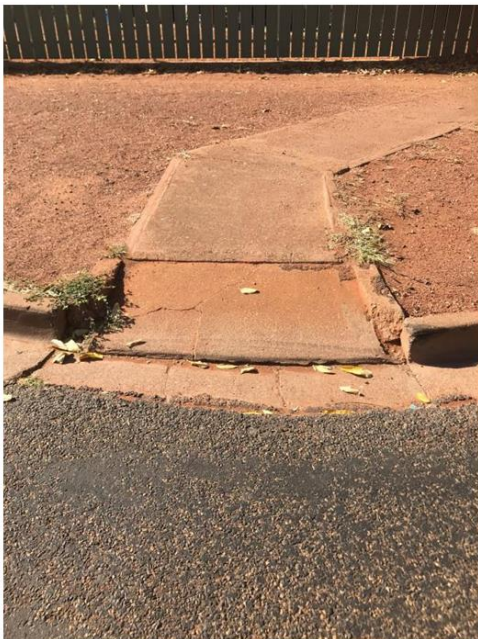
Point 10: Cat 1, reconstruct kerb ramp to size, shape and slope
