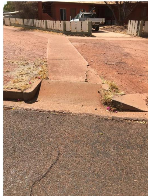
Point 20 : Cat 1, reconstruct kerb ramp and defective slab to size, shape and slope
