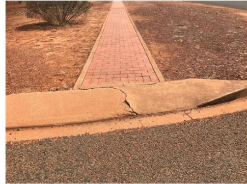
Point 27: Cat 2, correction of structural defect of the kerb ramp
