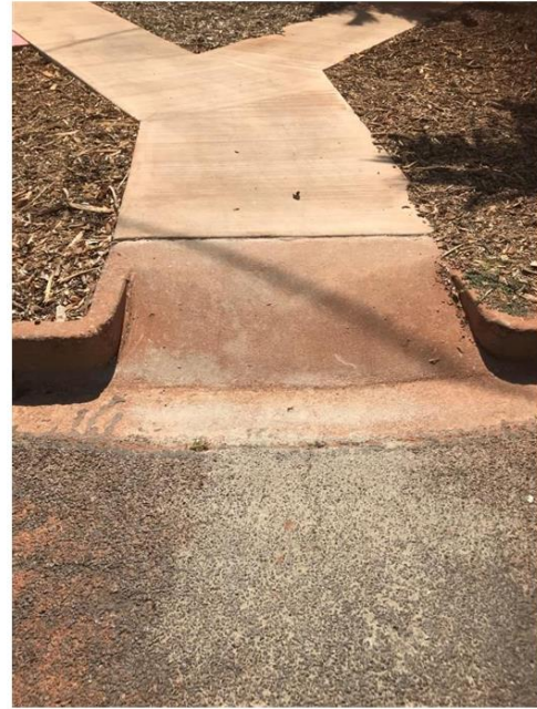
Point 19 : Cat 1, reconstruct kerb ramp to size, shape and slope
