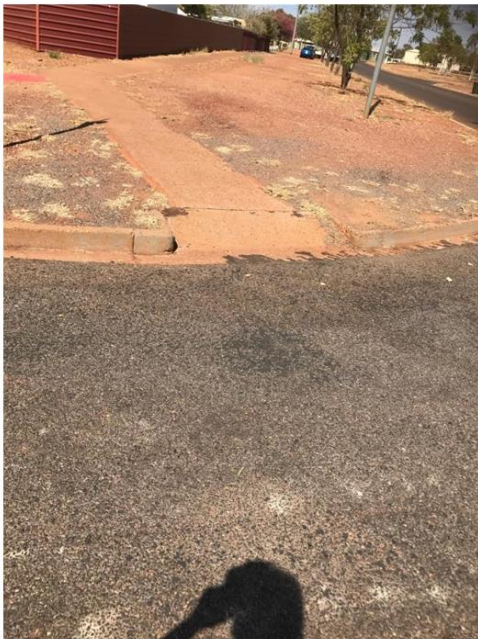
Point 18: Cat 1, reconstruct kerb ram to size, shape and slope
