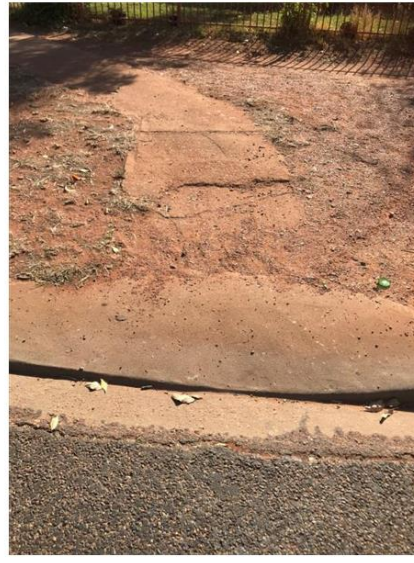
Point 2: Cat 1, reconstruct Kerb ramp to size, shape and slope including the reconstruction of approach slab.
