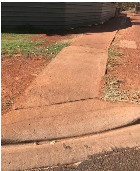
Point 3: Cat 2, reconstruct defective approach slab to size, shape and slope
