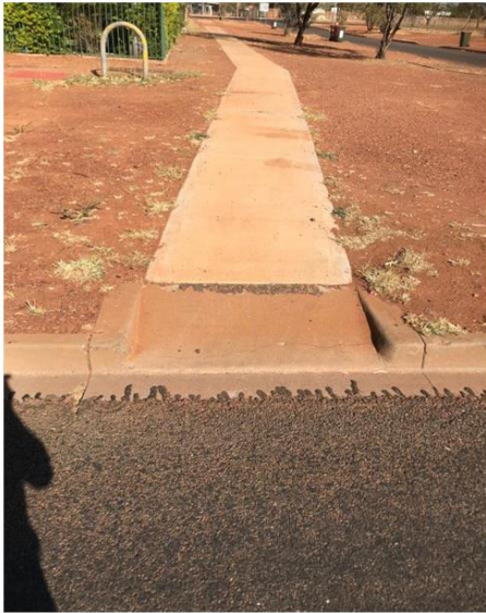
Point 1: Cat 1, reconstruct Kerb ramp to size, shape and slope.
