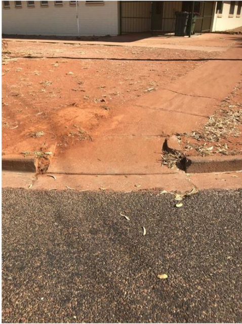
Point 9: Cat 1, reconstruct kerb ramp and defective slab to size, shape and slope
