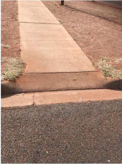
Point 13: Cat 1, reconstruct kerb ramp to size, shape and slope
