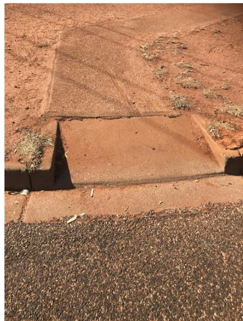
Point 12: Cat 1, reconstruct kerb ramp to size, shape and slope
