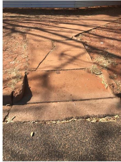
Point 7: Cat 1, reconstruct kerb ramp and defective slab to size, shape and slope
