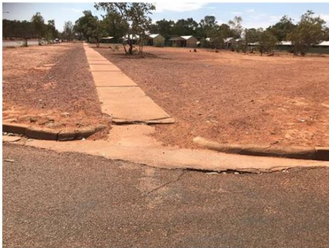
Point 26 : Cat 1, reconstruct kerb ramp to size, shape and slope
