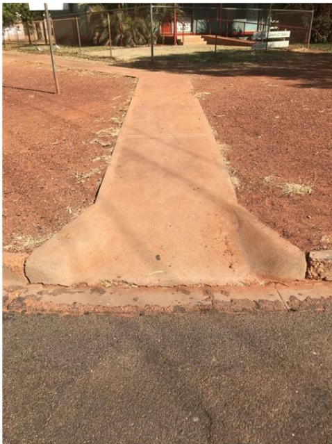
Point 14: Cat 1, reconstruct kerb ramp to size, shape and slope
