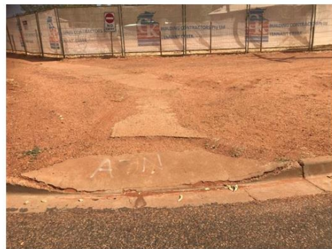
Point 24 : Cat 1, reconstruct kerb ramp and defective slab to size, shape and slope
