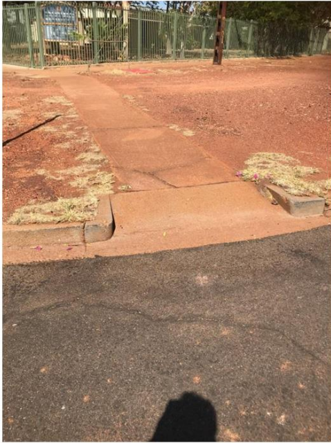
Point 21: Cat 1, reconstruct kerb ramp and defective slab to size, shape and slope
