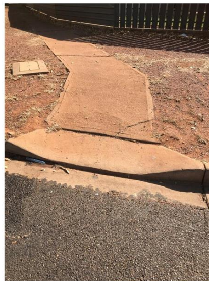
Point 4: Cat 3, grind the kerb ramp and approach slab to reduce the trip hazard
