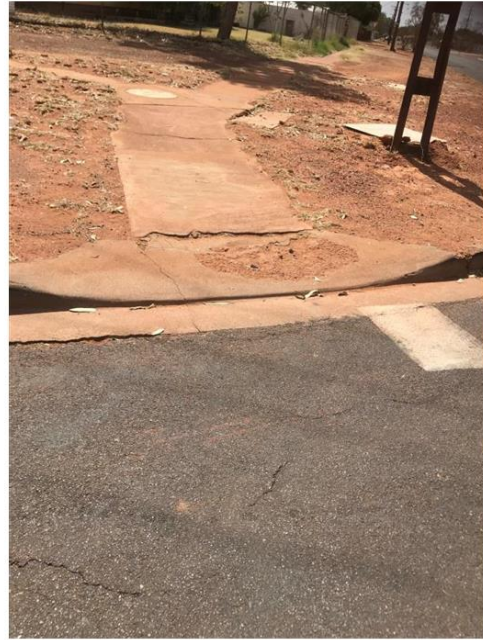
Point 23 : Cat 1, reconstruct kerb ramp to size, shape and slope
