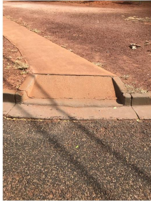
Point 15: Cat 1, reconstruct kerb ramp to size, shape, alignment and slope
