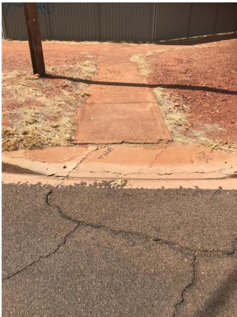
Point 22 : Cat 1, reconstruct kerb ramp to size, shape and slope
