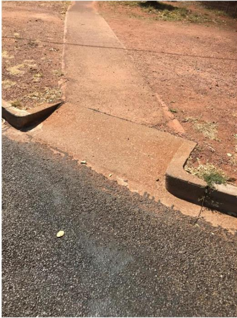
Point 17: Cat 1, reconstruct kerb ramp to size, shape and slope
