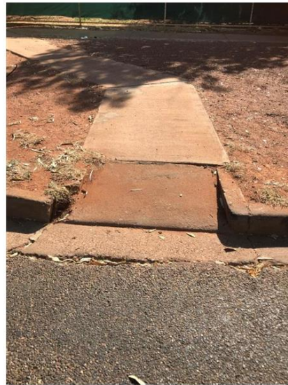
Point 8: Cat 1, reconstruct kerb ramp to size, shape and slope
