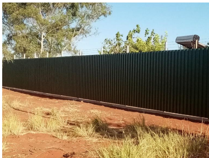
The new Ali Curung fencing – safe and secure. We have also applied for CCTV Camera’s and intercoms for both safe houses.
