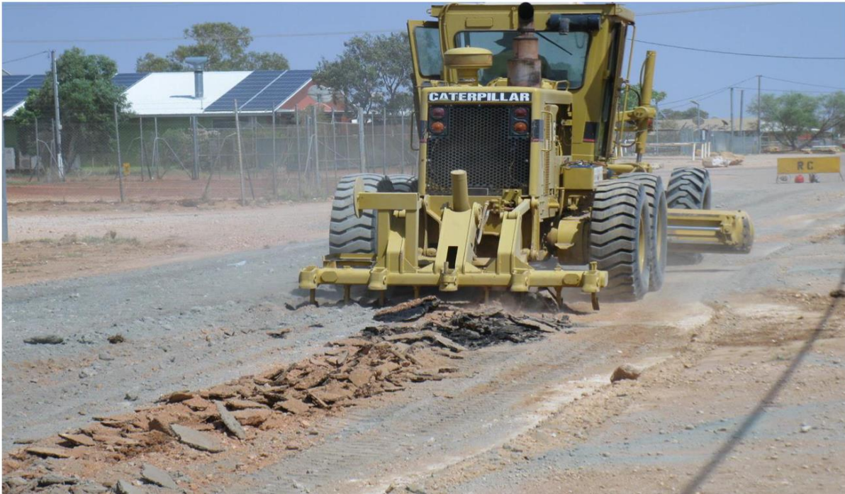
Top: Ripping of Antyiper St, Alpururulam; Bottom: Cement stabilization of Antyiper St
