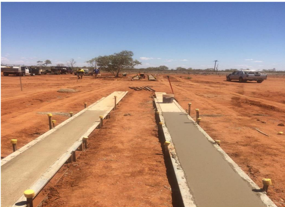
TC Cemetery – first double plinths (30 graves). Work awarded to Remote Concrete of TC.
